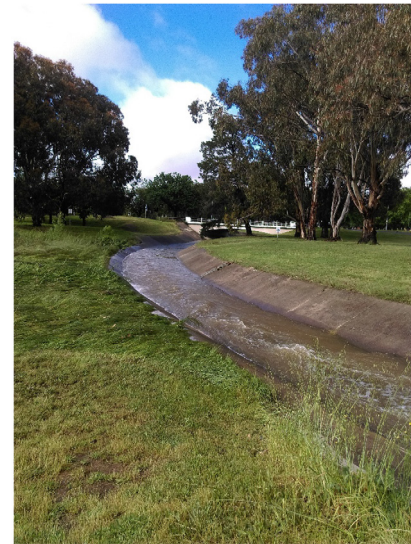
Fig. 7. Example of a concrete drain in northern Canberra, close to Lyneham Wetland, Australian Capital Territory, Australia.
